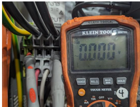
Figure 18: Image of de-energized charger. Digital multimeter is showing 0V across the ground cable (Green) and all 3 phases of the AC cable (Red, Black White).
