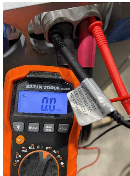
Figure 26: Image of de-energized Stromcore battery. The digital multimeter is showing 0V across the positive and negative cables at the discharge port.
